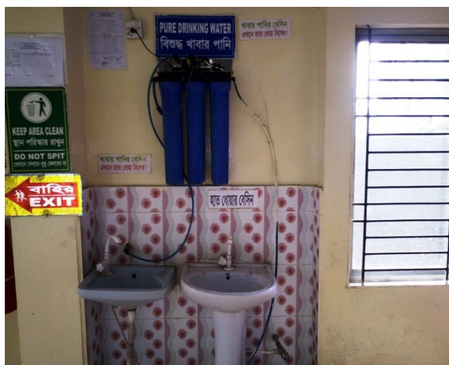
Pure Drinking Water Facility
